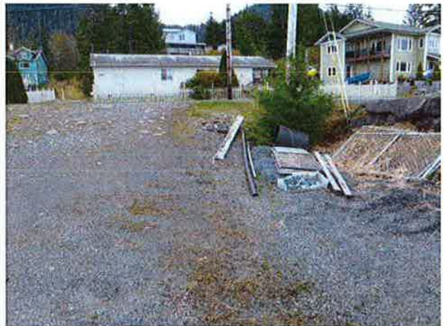
View from outlet across road to inlet. Culvert to be aligned to left of both power poles located in photo.
