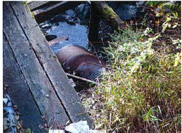
Outlet, structures surrounding with severe degradation of culvert visible. Outlet has steeper slope than inlet.
