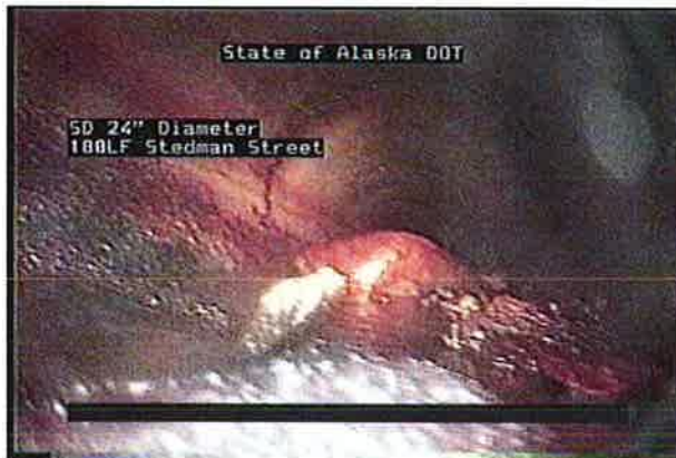
24-inch diameter, 100 feet reinforced concrete pipe (RCP). From video field notes: "Has lots of big rocks and humps in it that the vector truck can't pull out. Made it 15' in with camera no access to other side outfalls to beach." [sic]
