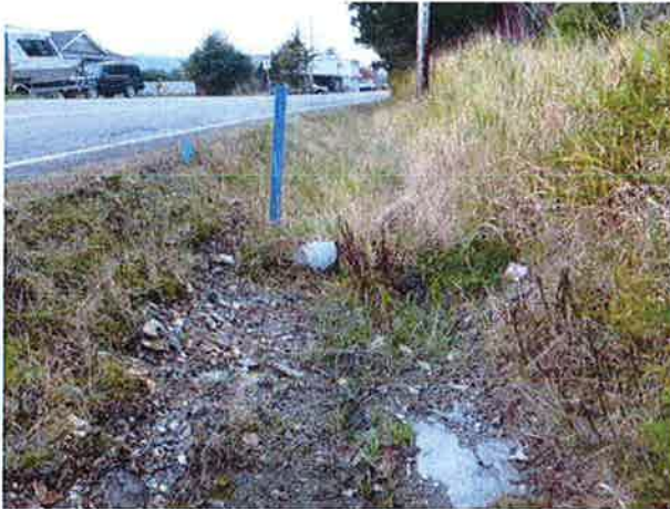
Inlet, erosion, and ditches looking north.
