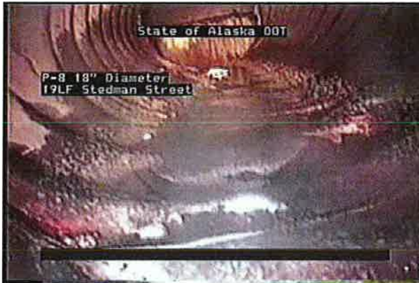
Corrosion and sediment in P-8.
