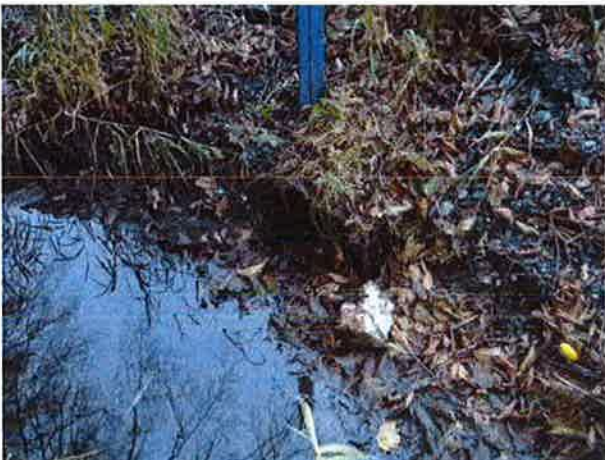
Ponding water at inlet; could indicate failure of culvert and water moving through road base.
