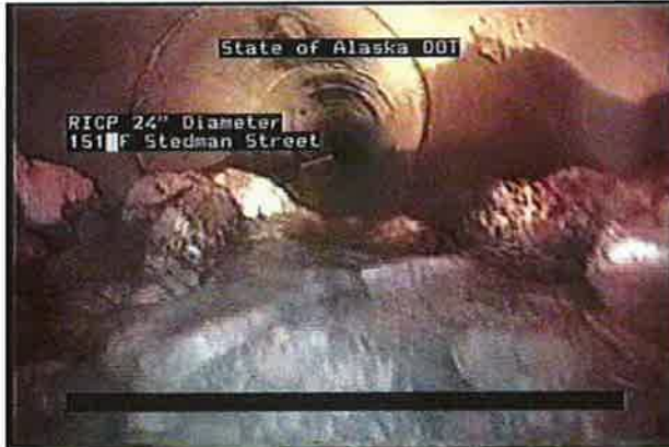
Large rocks and sediment inside pipe.
