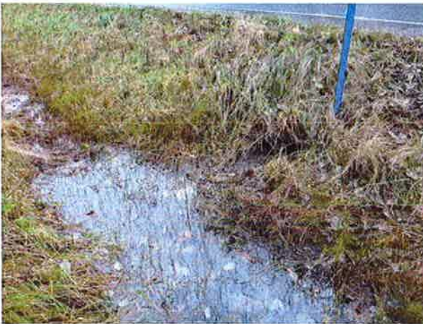
Ponding water at inlet.
