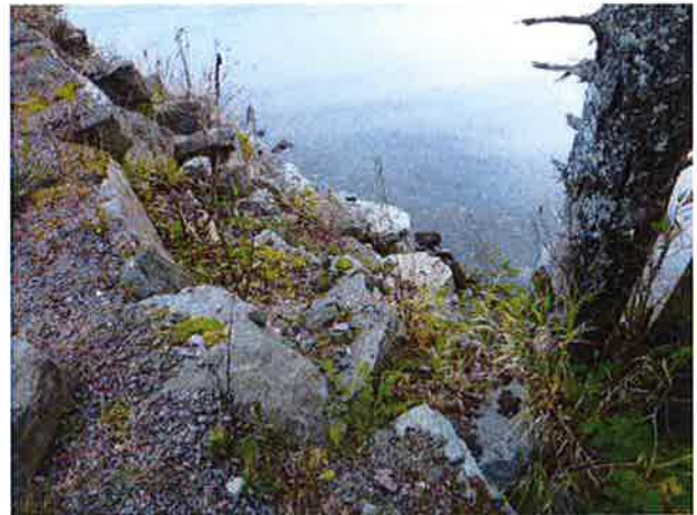
Rock retaining wall and fill have likely buried the outlet, as it was not found.
