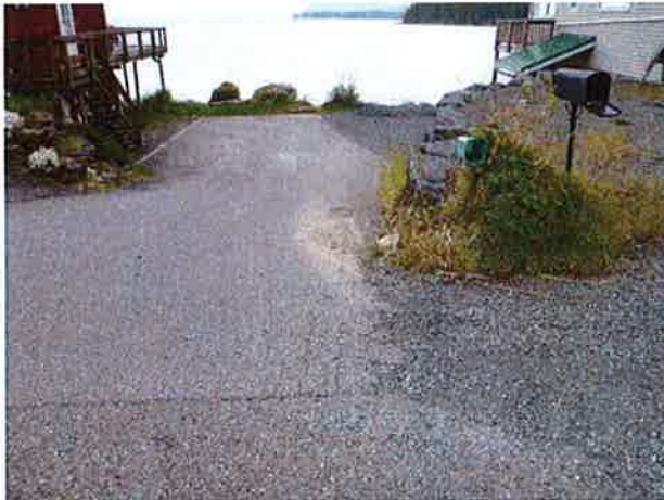
Alignment of culvert, moved south (left) by 10 feet to avoid rock retaining wall at photo right.
