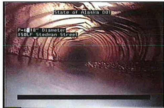
Structural failure and sediment in P-6.
