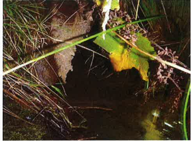
Close-up of inlet, severe corrosion visible.
