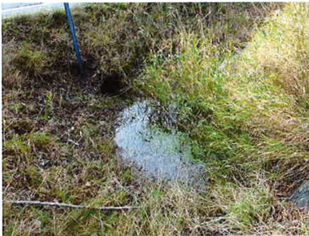
Ponding near inlet.
