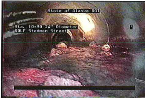
Rocks and sediment inside pipe.
