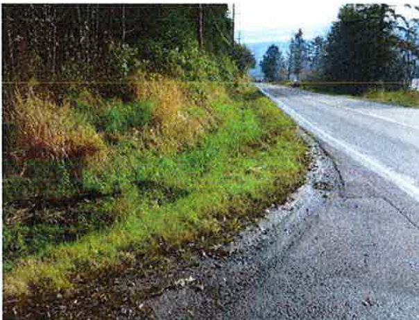
Propose combining with existing ditch to convey water to culvert at Station 146+51.
