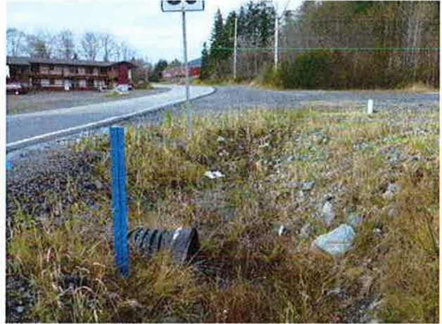
Ditch and parking area to the north. Asphalt being undermined due to lack of drainage path along road.
