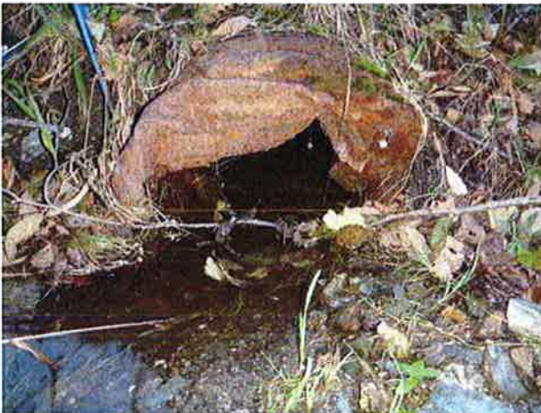
Damaged and corroded inlet.
