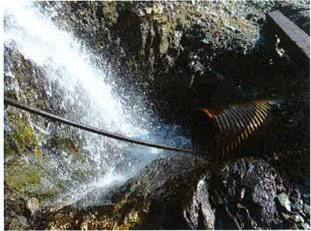
Inlet, with falls reaching culvert that was placed by removing bedrock. Parking area to photo right appears to experience erosion at high flows.
