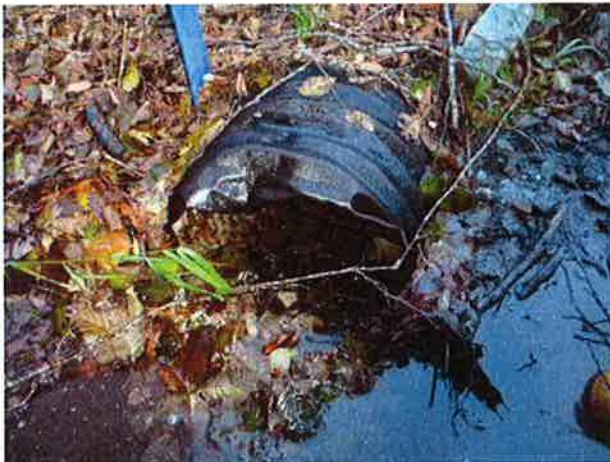
Inlet with standing water. Could indicate culvert failure and water moving through road base.
