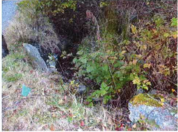
Inlet and property seep draining from north.
