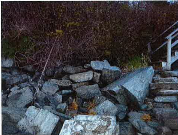
Location where water observed seeping from fill, likely location of outlet.
