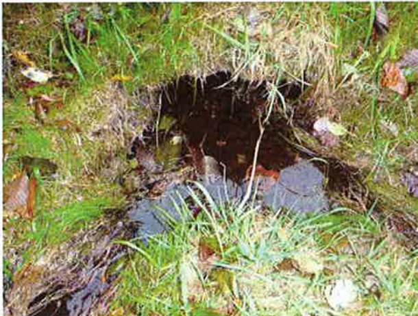
Inlet overgrown and partially buried.
