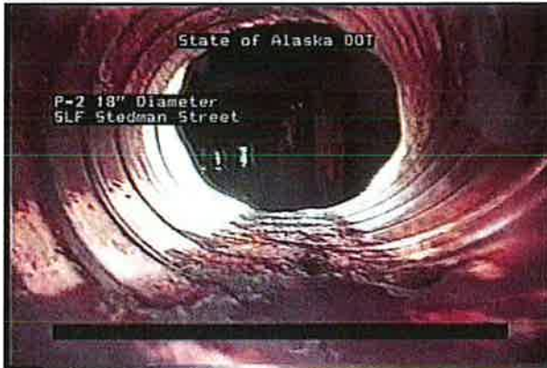
Corrosion inside pipe near outfall.
