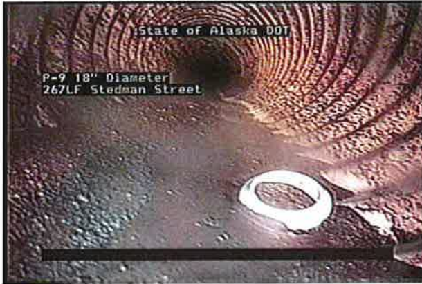
Corrosion, trash, and sediment in P-9.
