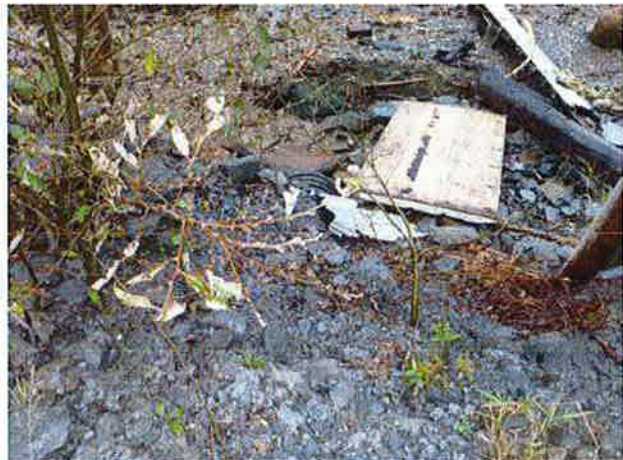
HDPE outlet at private property.
