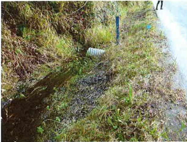
Inlet and ditches to south, ponding from water flow from north.
