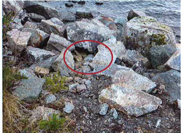
Culvert outlet crushed under fill.
