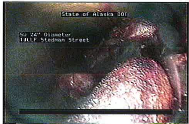
Large obstruction in pipe.
