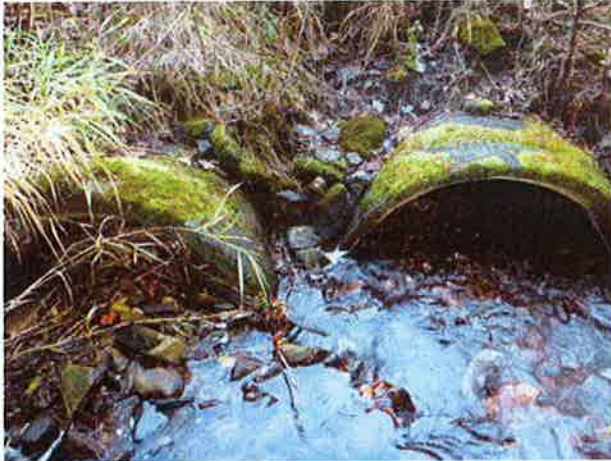
Inlet: Flow directed toward north barrel (photo right) as south barrel is clogged.
