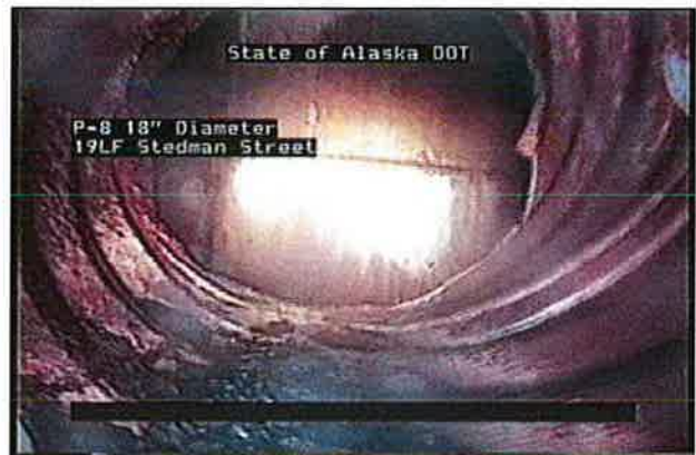
Corrosion and sediment in P-8.
