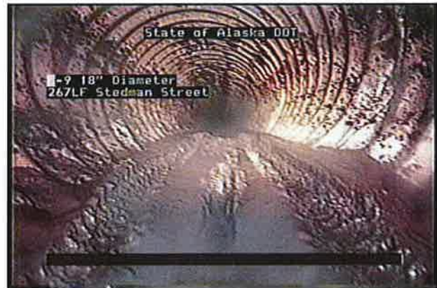
Corrosion and sediment in P-9.
