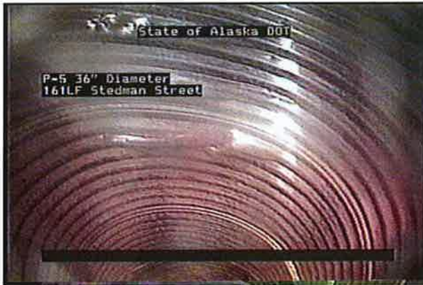
Structural failure in top of P-5.
