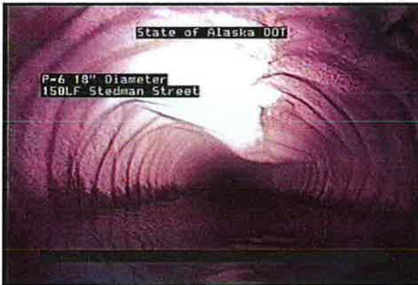
Pooling and structural failure in top of P-6.
