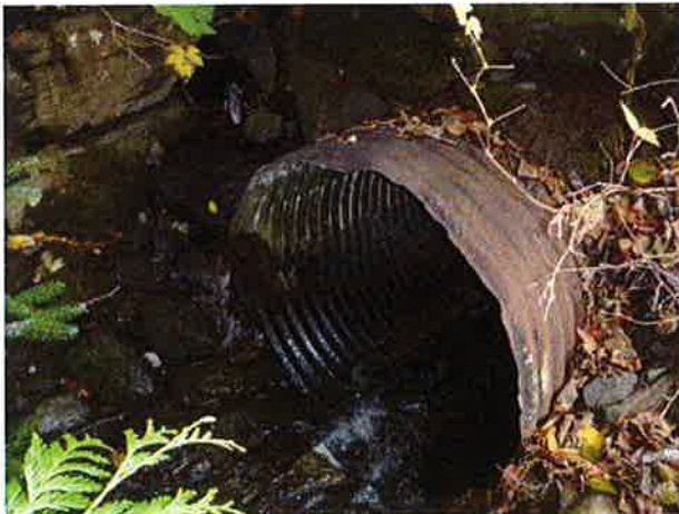
Inlet with corrosion.
