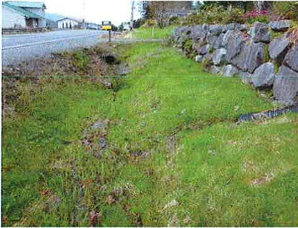
Inlet, driveway underdrain, and HDPE foundation drain discharge in view to north.
