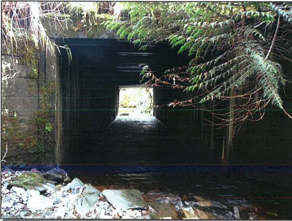
Site 032: Stream Crossing. Unnamed anadromous stream. Wooden box culvert. Photo taken October 15, 2015.
