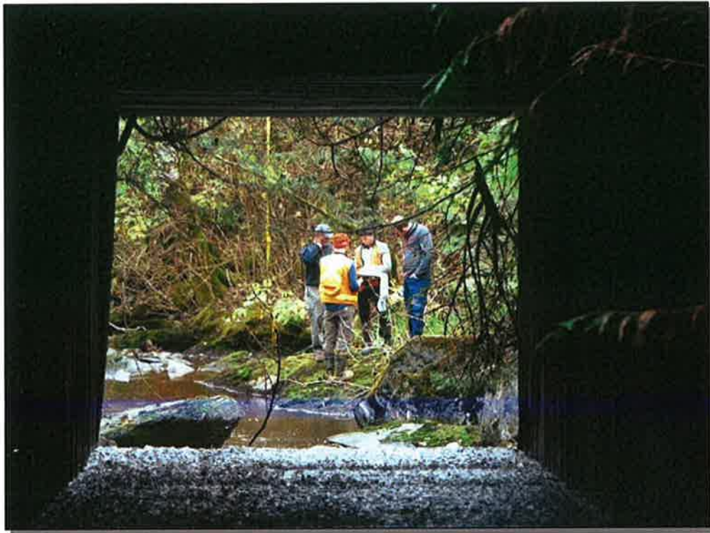
Site 032: Stream Crossing. Unnamed anadromous stream. Wooden box culvert. Photo taken October 15, 2015.
