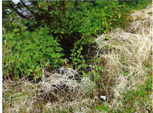
Outlet located on steep bank, incised channel, and causing erosion of road slope.
