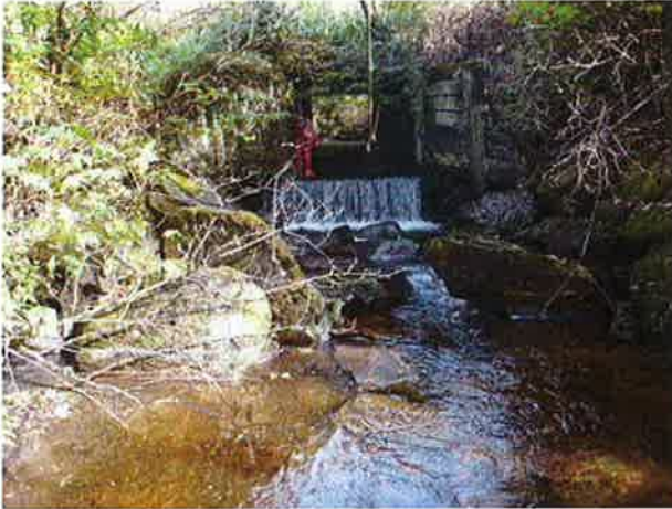
Outlet is a fish passage barrier with 3 feet between the invert and water surface downstream.
