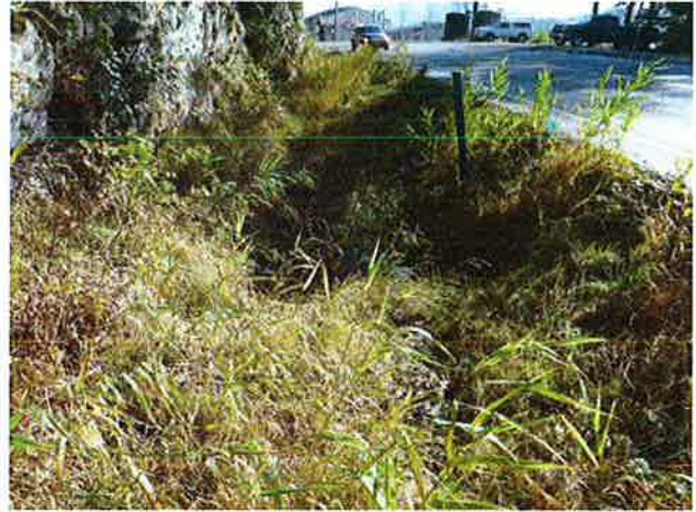
Ditches and bedrock outcrop to south of inlet. Inlet at blue post.
