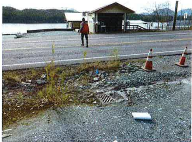
Alignment of culvert; directed toward house, under garage.
