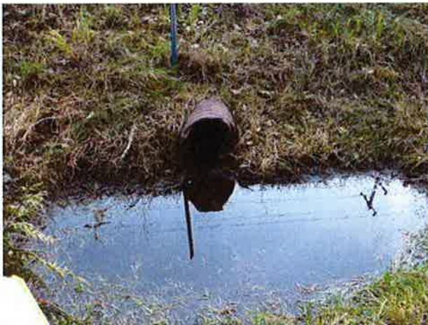
Inlet with ponding water.
