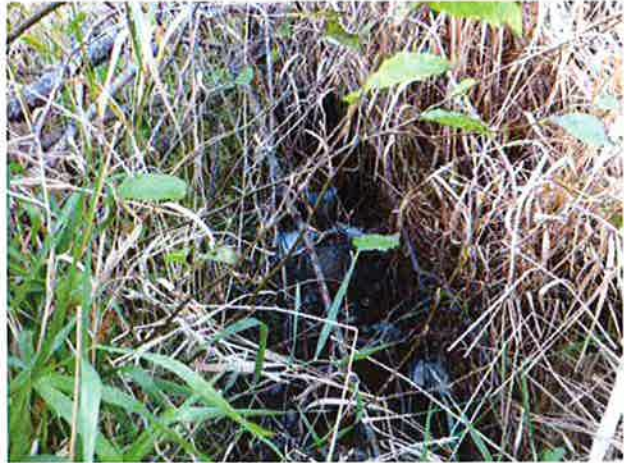
Outlet with incised channel, likely from low invert elevation and erodible substrate.
