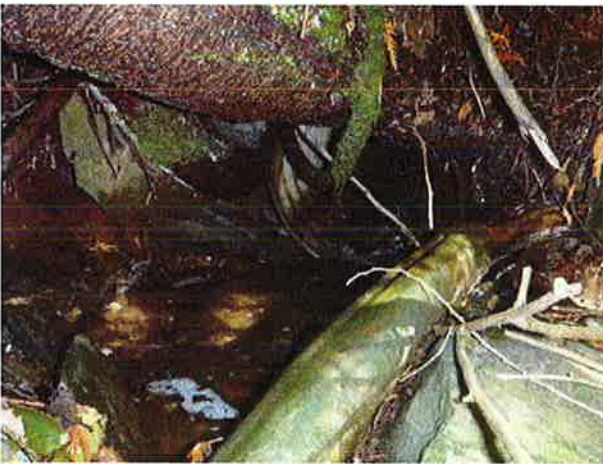
Outlet: Trees growing over top of outlet.
