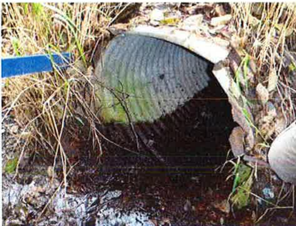
Inlet. Corroded invert.
