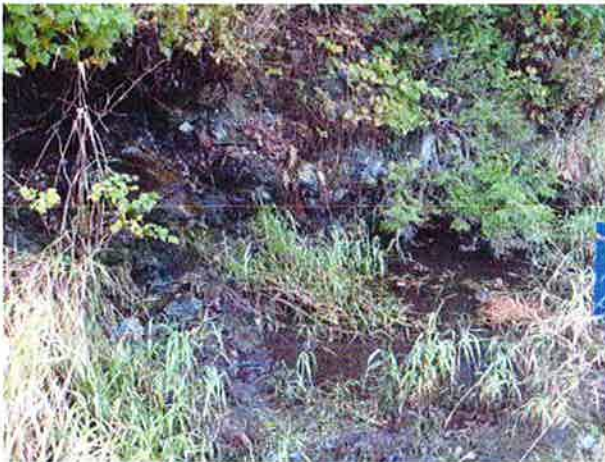
Seep and ponding water at inlet.
