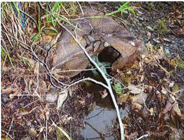
Crushed and corroded inlet.
