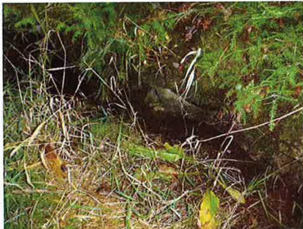
Outlet: South barrel clogged at outlet, north barrel (photo left).
