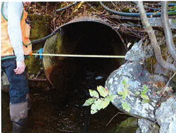
Outlet with HWM visible.
