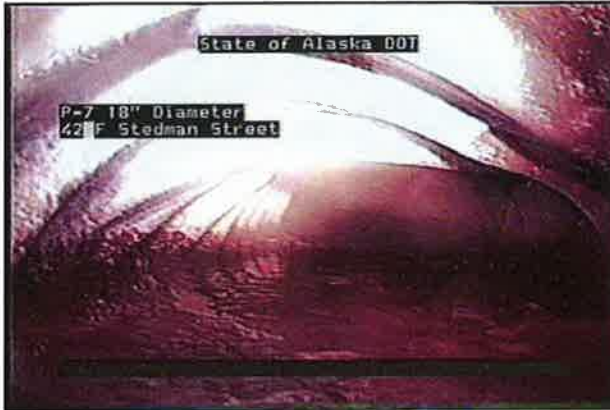
Sediment and structural failure in top of P-7.
