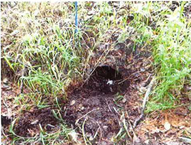
Inlet partially buried and corroded.
