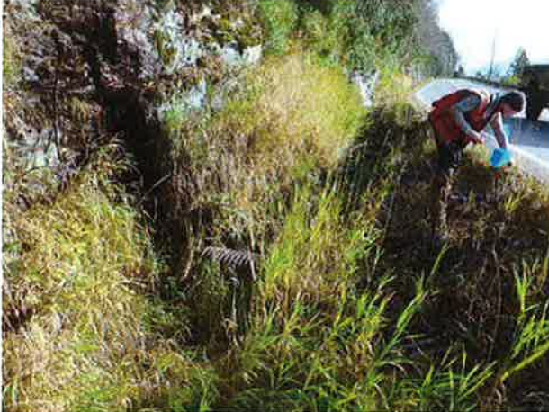
Ditches to south of inlet. Possibly direct flow through this ditch to culvert at Station 70+21.
