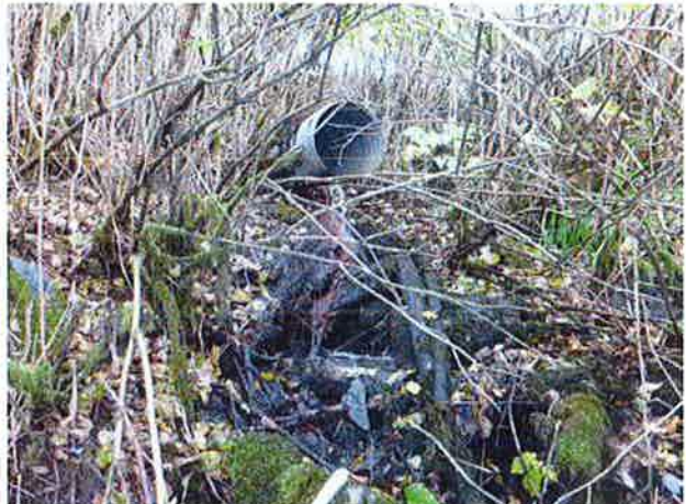
Current outlet with discharge present.
