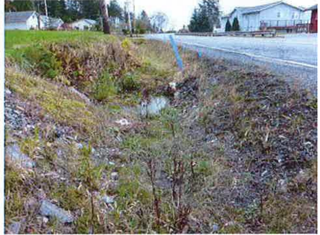
Inlet and ditches to south. Erosion and evidence of backwater at inlet visible.
