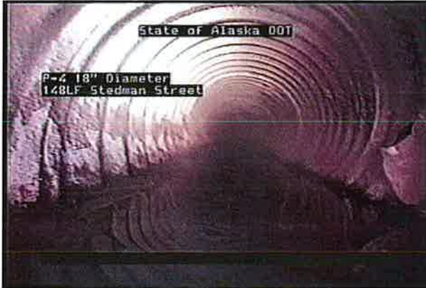
Rupture in side of P-4.
