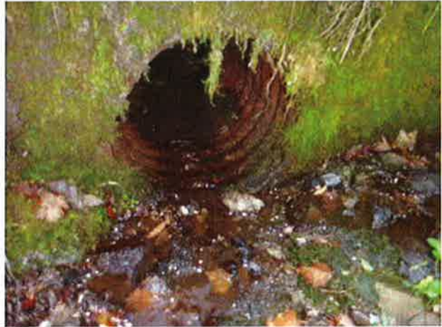
Concrete headwall at inlet. Note invert missing from culvert.
