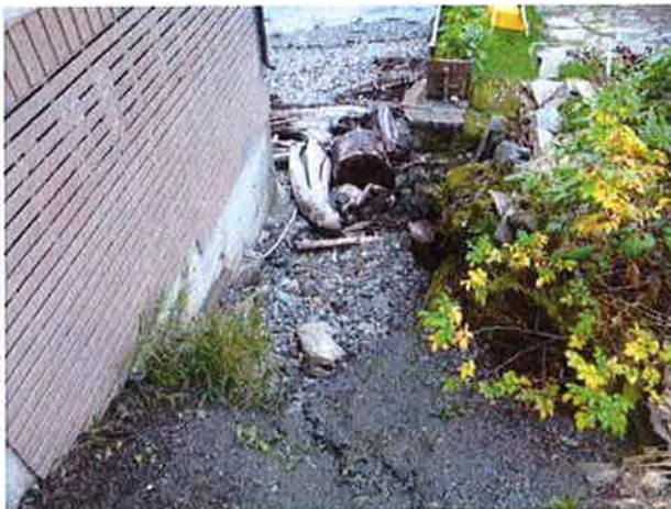
Outlet discharging adjacent to house foundation.
