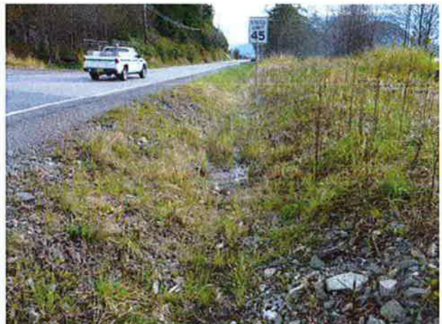
Existing outlet filled with sediment; low slope ditch conveys water to south along highway.
