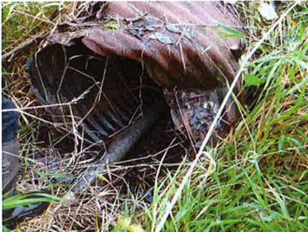
Inlet. Damage and corrosion present with 4-inch steel pipe running through culvert.
