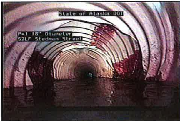
Corrosion and buckling inside pipe.
