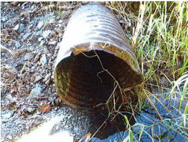
Inlet with corrosion and damage.
