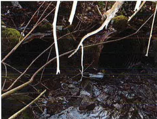
Double barrel inlet, corrosion and damage visible.
