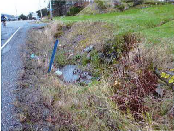
Inlet with ponding at inlet, view north. Incised ditch from property foundation drain at right of photo.
