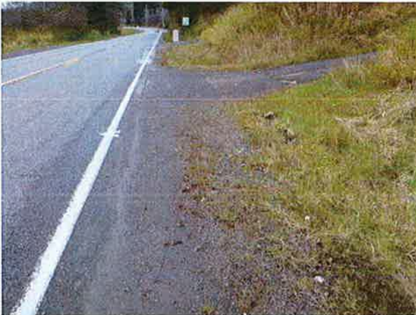
Distance view of inlet near mailbox, two driveway crossings, and grading of ditch to direct water south.
