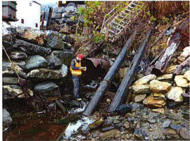
Outlet. Highly corroded with pilings and debris nearby.
