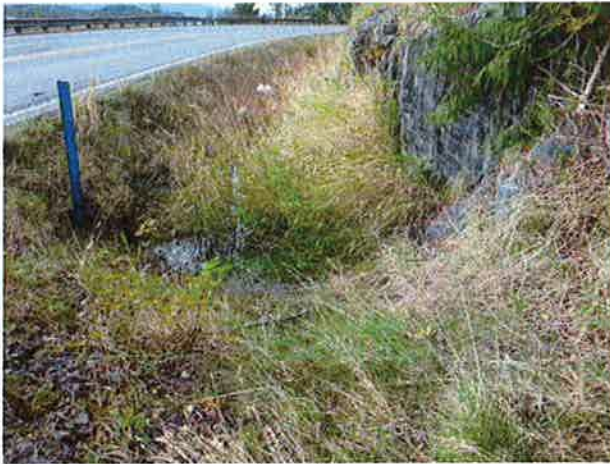
Inlet and ponding visible at blue marker. Ditches to north.
