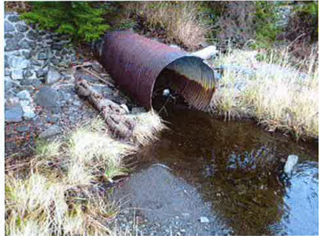
Outlet at high tide line, invert corroded away.
